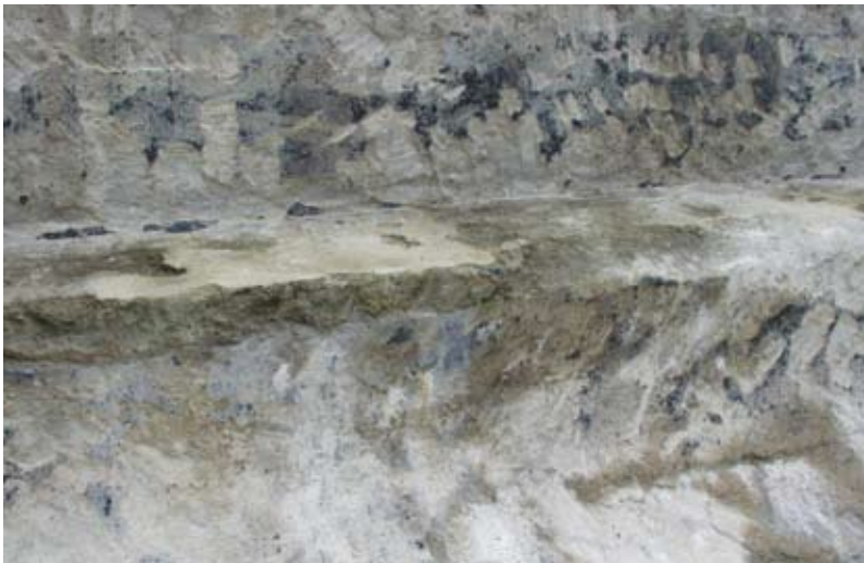
Evidence of the use of rebound often shows up years later, when a pool's interior plaster is stripped for refinishing. In all of these cases, the rebound-bearing steps and benches fell apart once the plaster that held them together was removed, leaving the homeowners and plasterers with messes that won't just take care of themselves, and the pool construction industry with a black eye it really doesn't need
